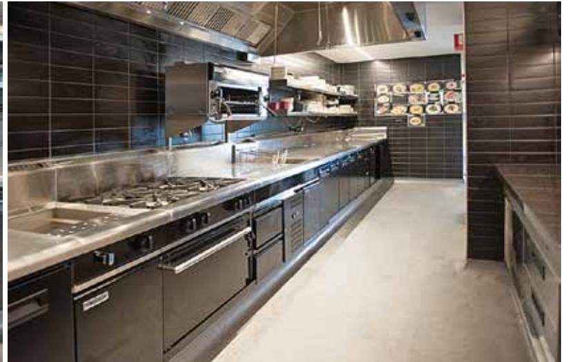
PROJECT SUPPLIED BY HILL EQUIPMENT, SOUTH AUSTRALIA
