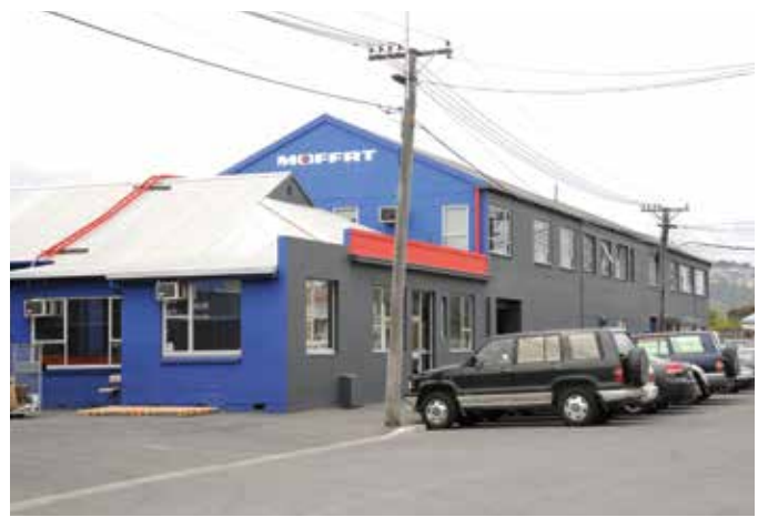
ABOVE IS THE OSBORNE STREET FACTORY DAMAGED IN THE EARTHQUAKES OF 2010 AND 2011
